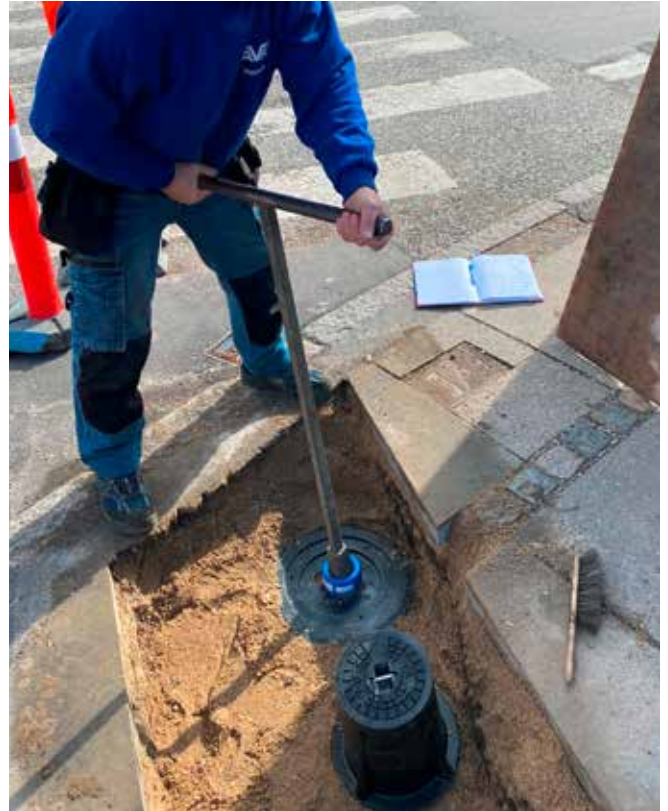
Underground gate valve with VIDI Positioner that detects when the valve is operated.
