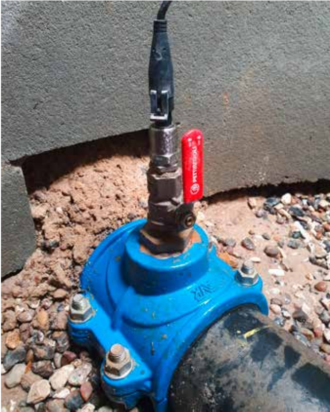
Due to the wireless nature of IoT, the pressure sensors can be installed at any critical point in the distribution network.
